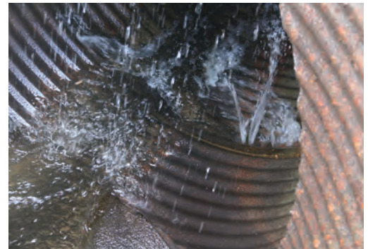
Water jets into the outlet pipe in the dam at Pibel Lake Recreation Area. The LLNRD plans to begin replacement of the outlet pipe in December.
