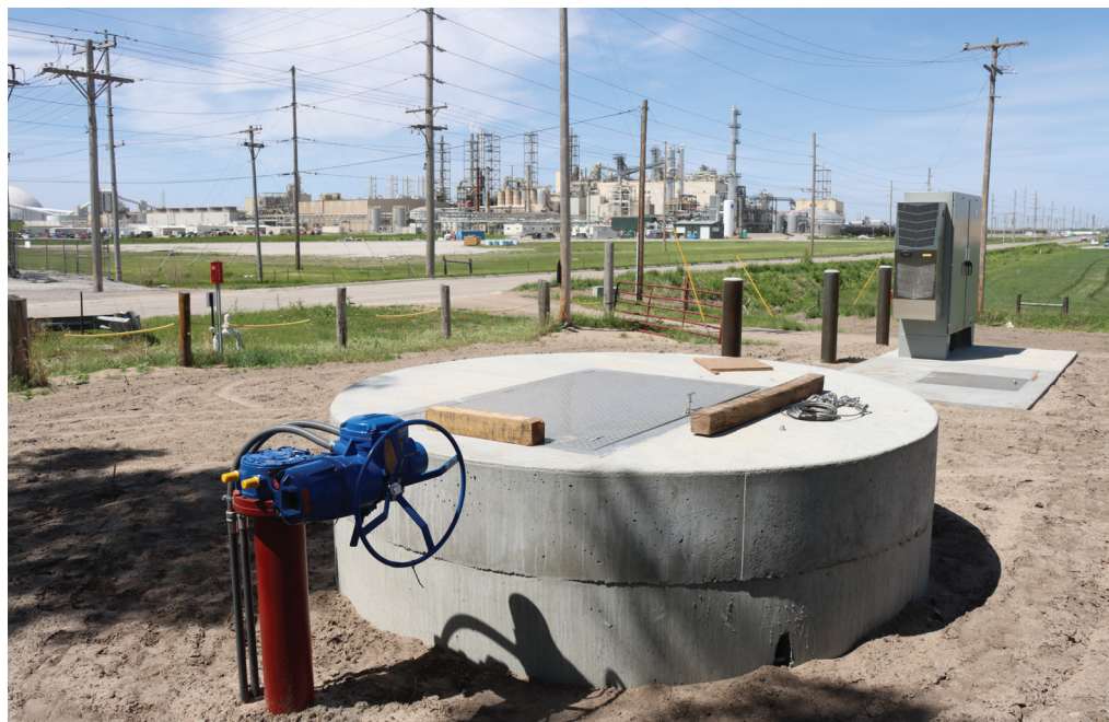
The main pump station for the Columbus Area Recharge Project is located on Eighth Street in Columbus.
